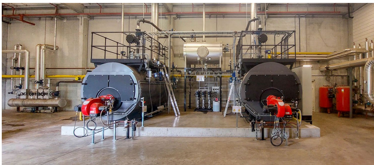
2 steam boilers of 5 T/h in cascade arrangement, with high-efficiency degasser
