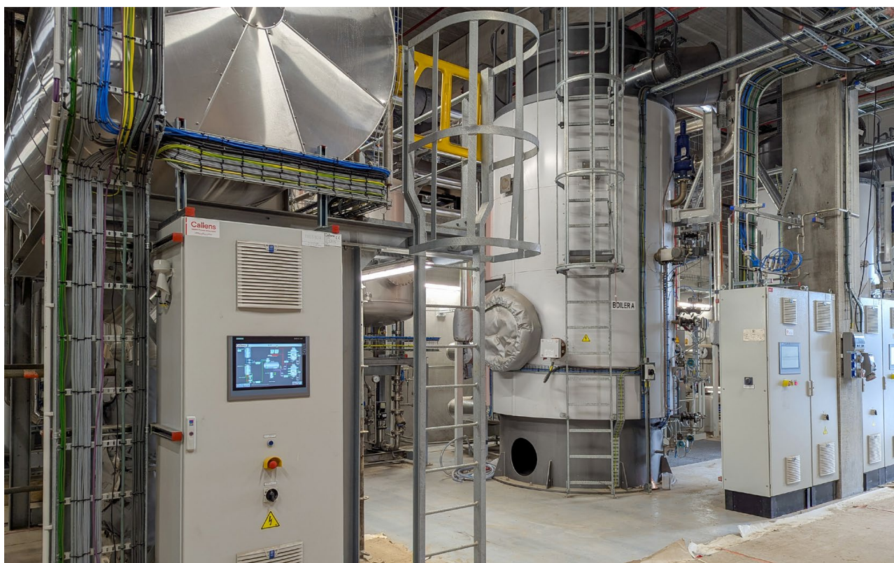
2 e-boilers, each with a capacity of 5 MW and 7.5 T/h steam, including balance of plant
